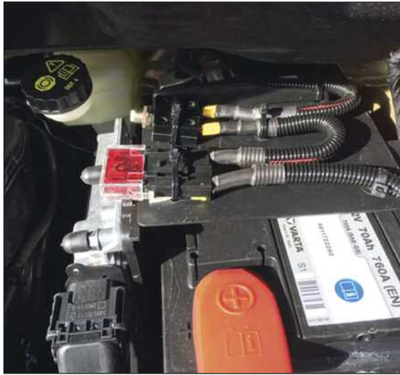
Figure 26 – Accessible Berlingo Fuse and Thermal Cut Out Switch.
