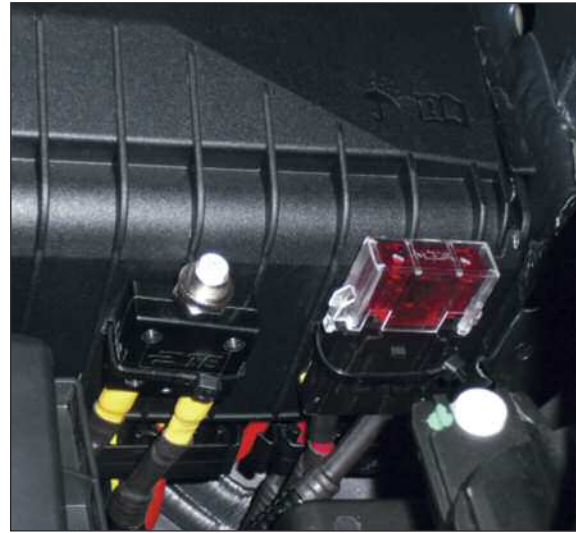
Figure 27 – Accessible Maxi Fuse and Thermal Cut Out Switch.
